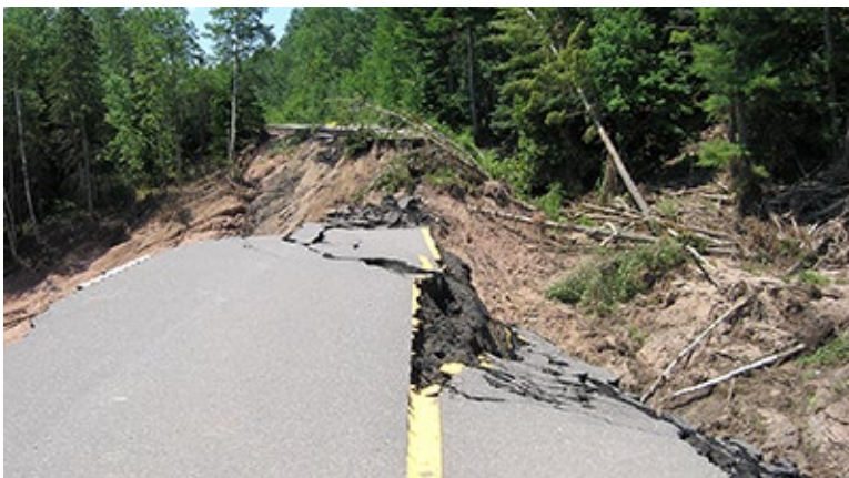
Figure 1. Highway 210 flooding damage (Photo Credit: Jim Sorenson)
